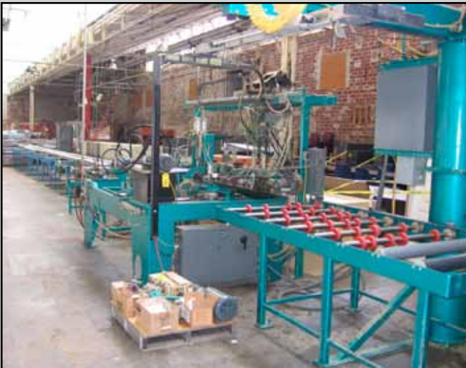
(1 OF 2) KVAL 990 DOOR MACHINES—REAR VIEW
